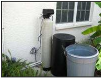
6.0 Picture 1 Conditioning system North wall
