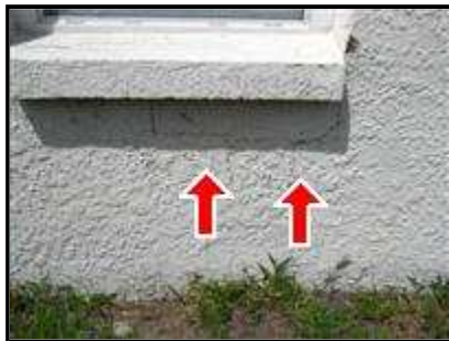
2.1 Picture 5 Crack under other window, South side
