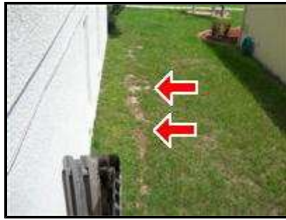
1.2 Picture 5 .... causing erosion here.
