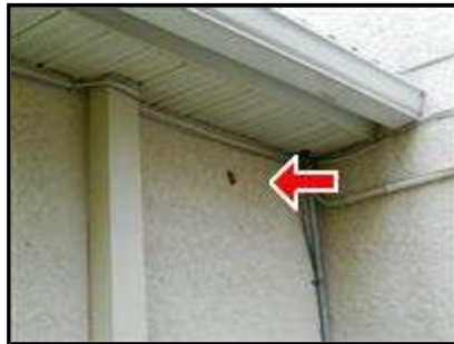
2.9 Picture 9 At AC compressor
