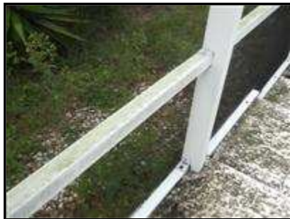
12.23 Picture 7 Pool cage needs pressure wash too.
