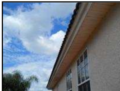
1.2 Picture 2 Recommend roof drainage system on upper level of West side....
