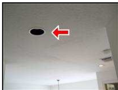
7.4 Picture 7 Top story hallway - bulb expired.
