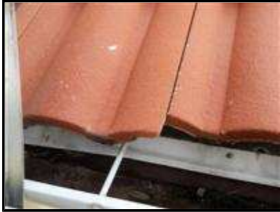
1.1 Picture 4 Tiles have moved over gutter.
