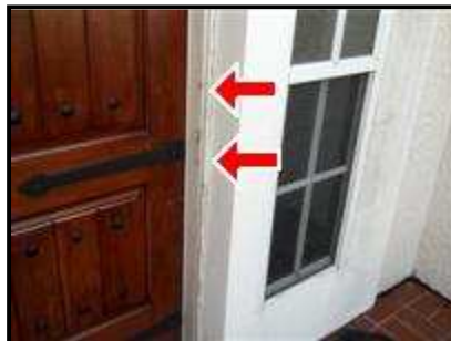
2.2 Picture 1 Door frame needs painting.
