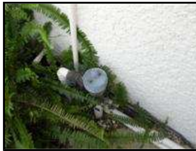
11.1 Picture 1 Sprinkler controller on right side.
