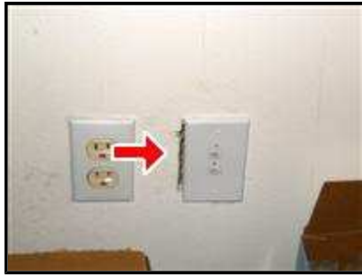
4.2 Picture 13 Seal gap - den.
