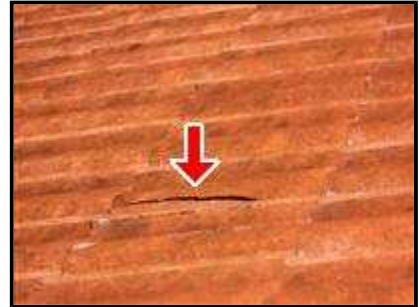
1.1 Picture 18 Minor cracked tile over lower West side.
