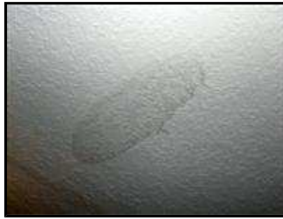
4.1 Picture 1 Ceiling stain in living room - paint.
