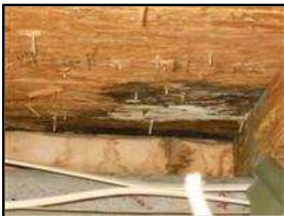
1.1 Picture 10 Damage to roof sheathing under affected area.
