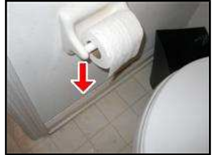
4.3 Picture 6 Baseboard separating from wall in toilet room adjacent to the tub in previous picture.
