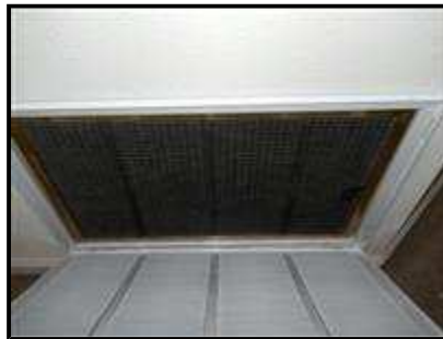
8.1 Picture 5 Washable filter on top floor will need washing soon
