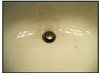
6.2 Picture 3 Corroded drain hardware - master
