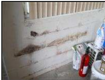
3.2 Picture 1 Wall at window bumpout in garage is stained. No active leak was detected and the meter read normal when tested. Patch,
