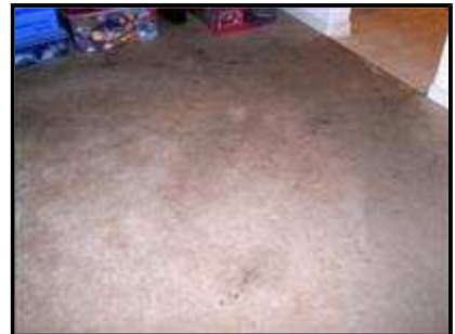
4.3 Picture 12 Stained carpet - dining room
