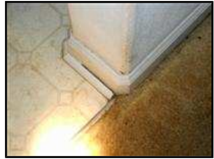
4.2 Picture 15 Repair baseboard trim at kitchen entry.
