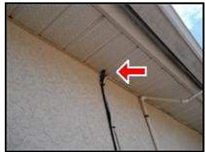
2.8 Picture 3 Seal gap - right of garage.
