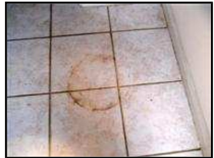
4.3 Picture 9 Stained tile - front entry
