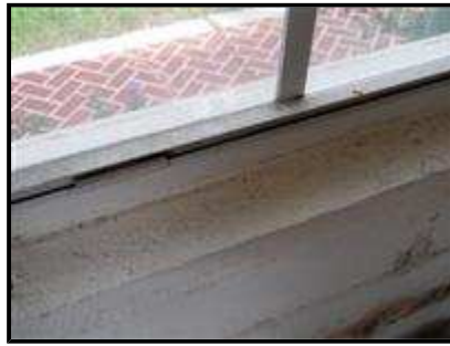
2.3 Picture 2 Same window does not latch well.
