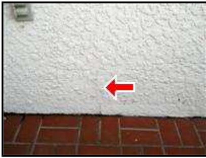
2.1 Picture 11 Crack right of front entry at garage wall.
