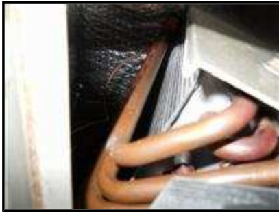
8.1 Picture 1 Unit # 1 in garage
