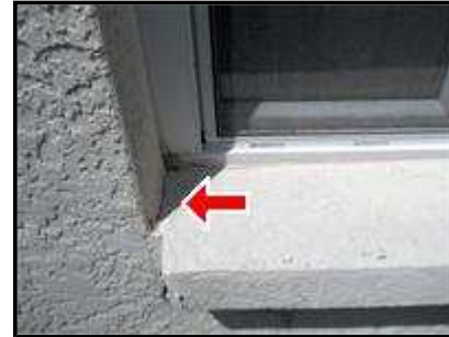
2.1 Picture 4 Seal gap at sill, South side
