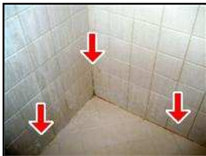
4.2 Picture 7 Clean, repair and/or caulk needed in master shower.
