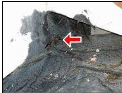
1.1 Picture 8 Deteriorating underlayment and tar.
