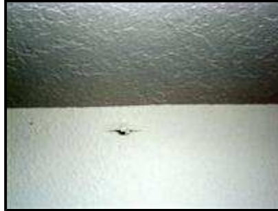
3.2 Picture 4 Nail pop - near door to laundry in garage.
