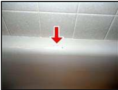
6.2 Picture 1 Chipped tub - Upstairs guest bath.
