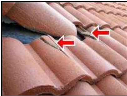
1.1 Picture 7 Cracked tiles and exposed underlayment.
