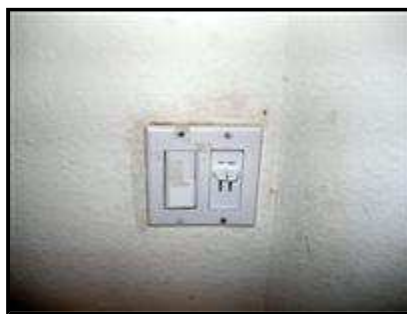
7.4 Picture 5 Switch in master appears damaged, replace as necessary.
