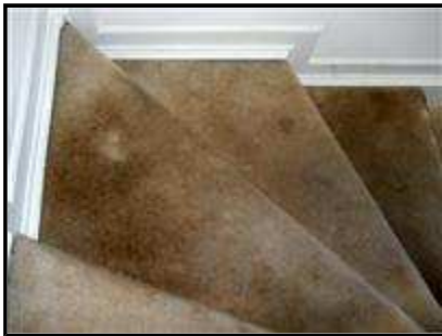
4.3 Picture 7 Stained carpet on stairs
