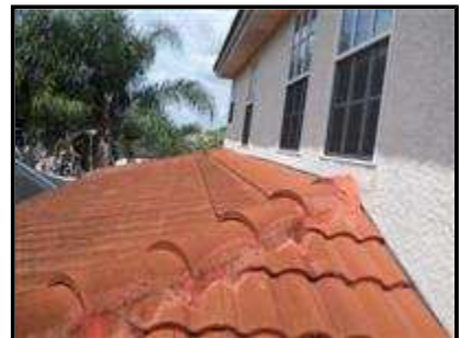
1.2 Picture 3 ... causing staining on lower section over patio.
