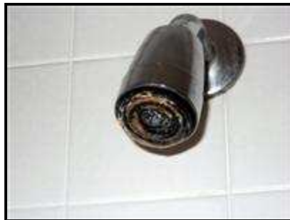
6.2 Picture 4 Corroded shower head in master.
