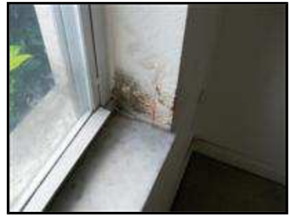
4.2 Picture 12 Den window opening is stained.
