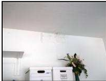
3.2 Picture 2 Stain from leak in roof explained in roofing section.
