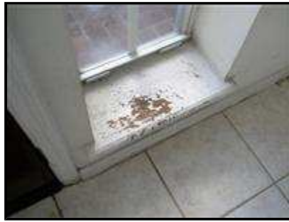
4.2 Picture 11 Wood window sill at front entry door needs repair and paint.
