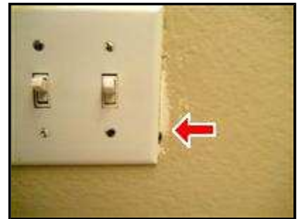
4.2 Picture 6 Seal gap at light switch - master bath
