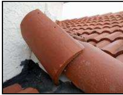
1.1 Picture 2 Same tiles in previous picture - loose from fasteners and grout.
