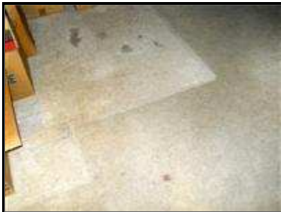
4.3 Picture 10 Stained carpet in den.
