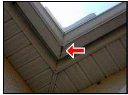
1.2 Picture 6 Seam leak over front entry
