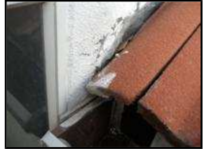
1.1 Picture 6 Area next to wall needs to be further inspected and sealed as necessary.
