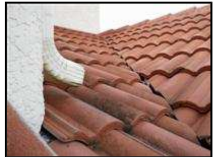
1.1 Picture 9 Downspout from upper level drains onto this affected area.
