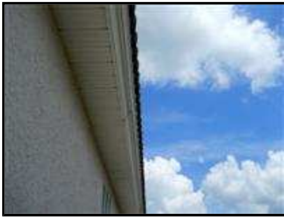
1.2 Picture 4 Lack of upper gutter here....
