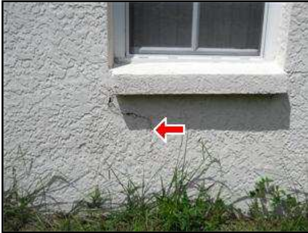
2.1 Picture 3 Step crack, South side, lower story
