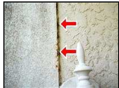
2.1 Picture 10 Patch & paint - right of front entry.
