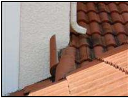
1.1 Picture 1 To right of front entry over garage.
