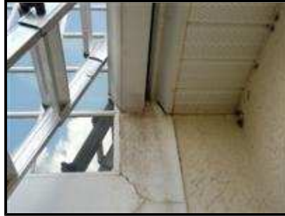
1.1 Picture 5 Stains from leak above.
